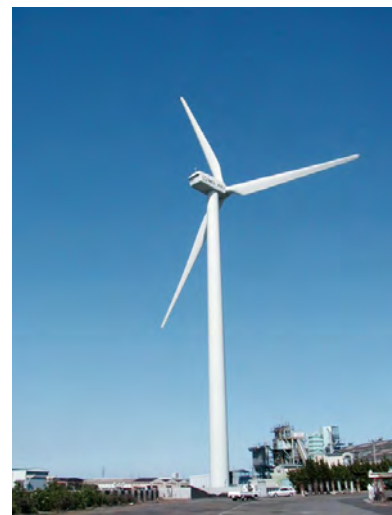
Ichihara Wind farm ( MJ Wind power Ichihara CO., LTD. ) Ichihara City, Chiba
