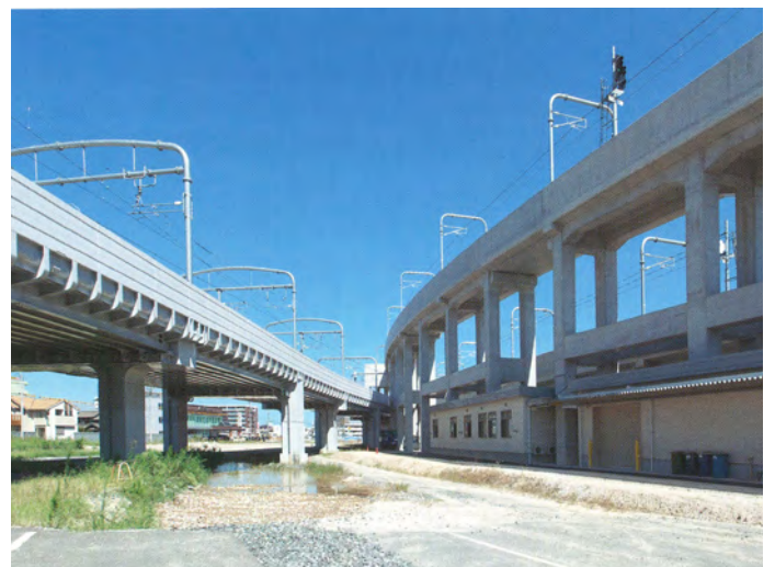
Railway-road continuous grade separation project for Otagawa Station of Tokoname Line / Kowa Line and neighboring area Ota-machi and Takayokosuka-machi, Tokai City Completion:2011
